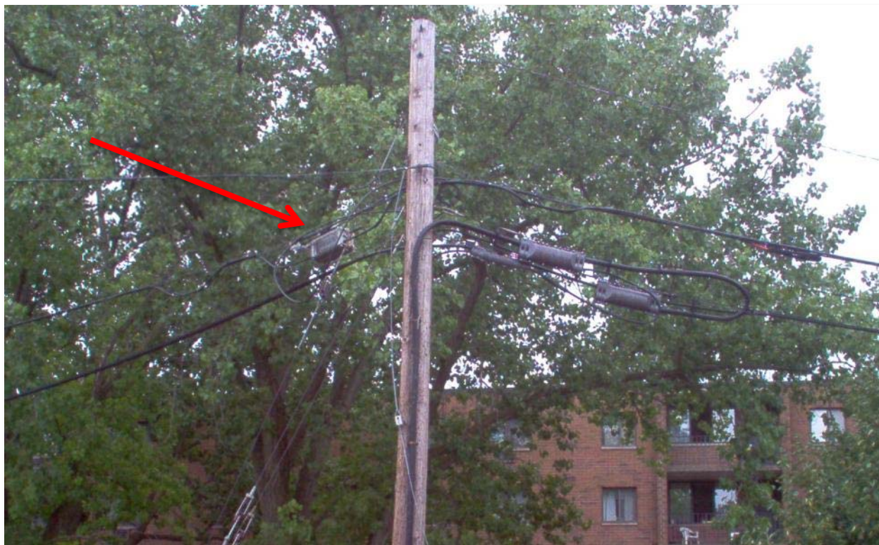
Figure 15: Utility Pole with Cable Amplifier
