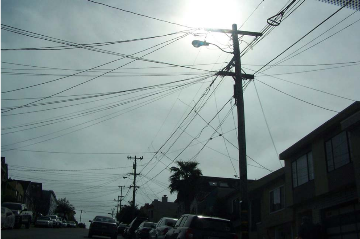
Figure 2: Crowded Utility Pole Line in Bayview
