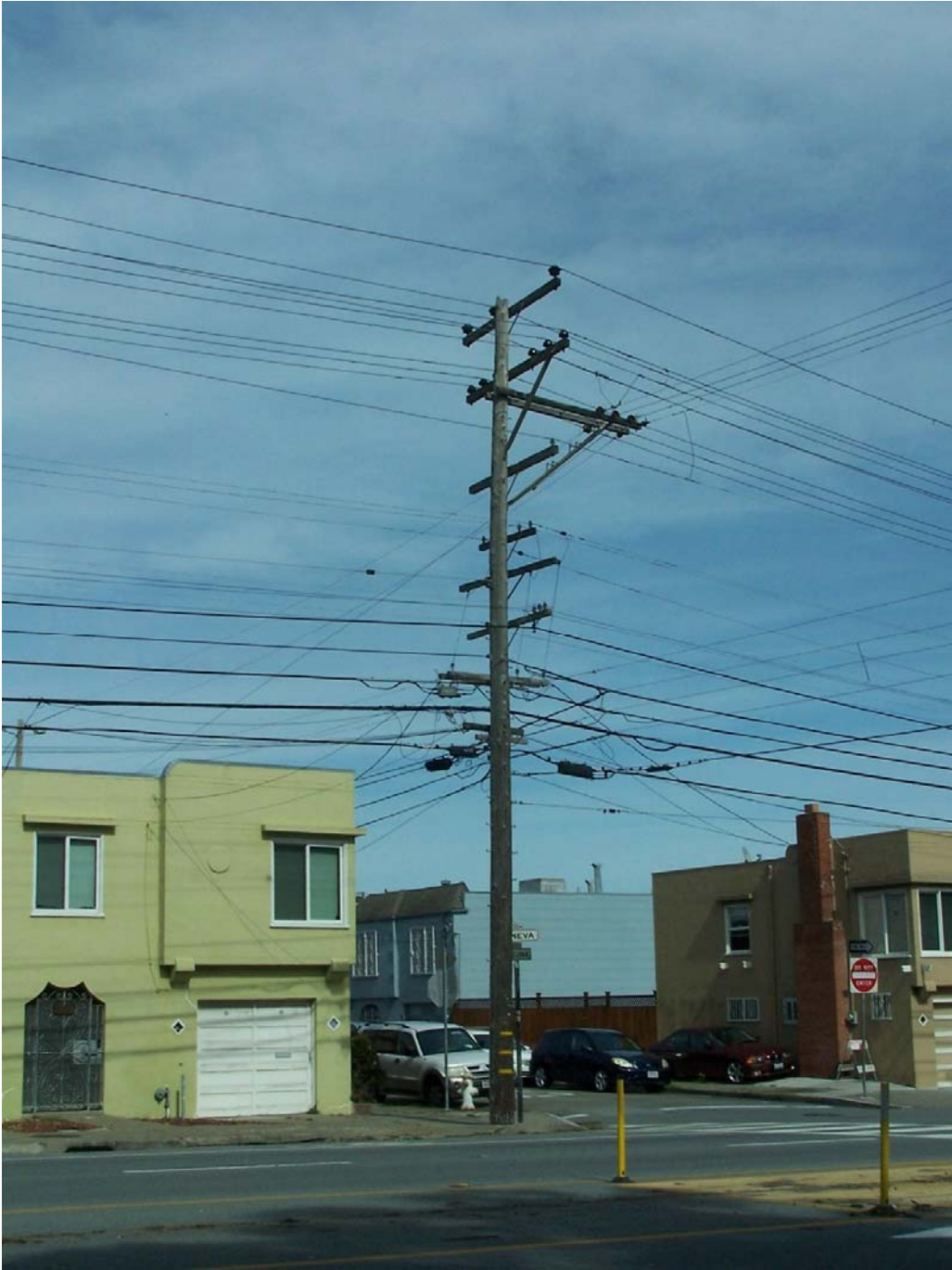
Figure 3: Utility Pole Requiring Make-Ready in Excelsior
