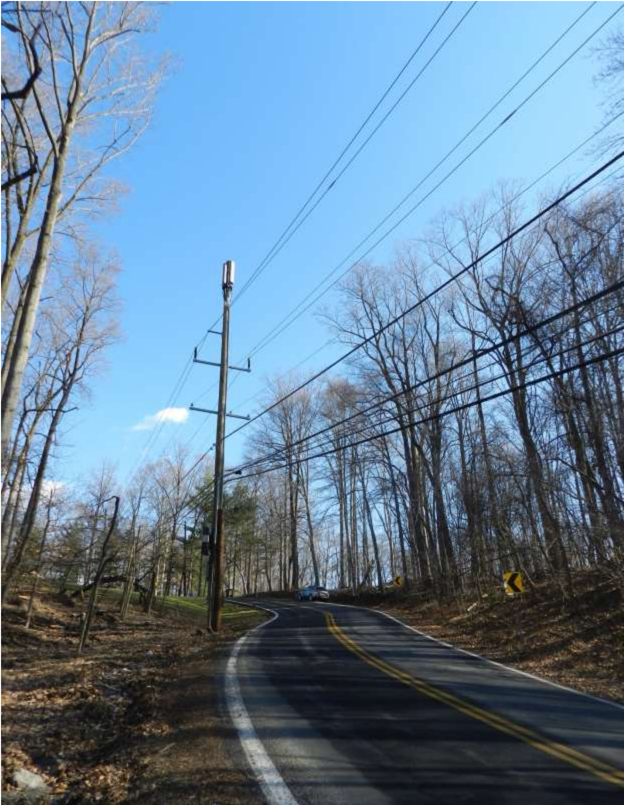
Figure 6—Small Cell at Height of High Voltage Transmission Lines
