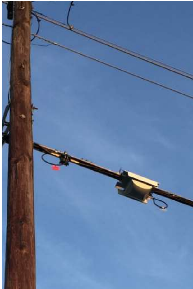
Figure 9 – Wi-Fi Antenna on Cable TV Attachment
