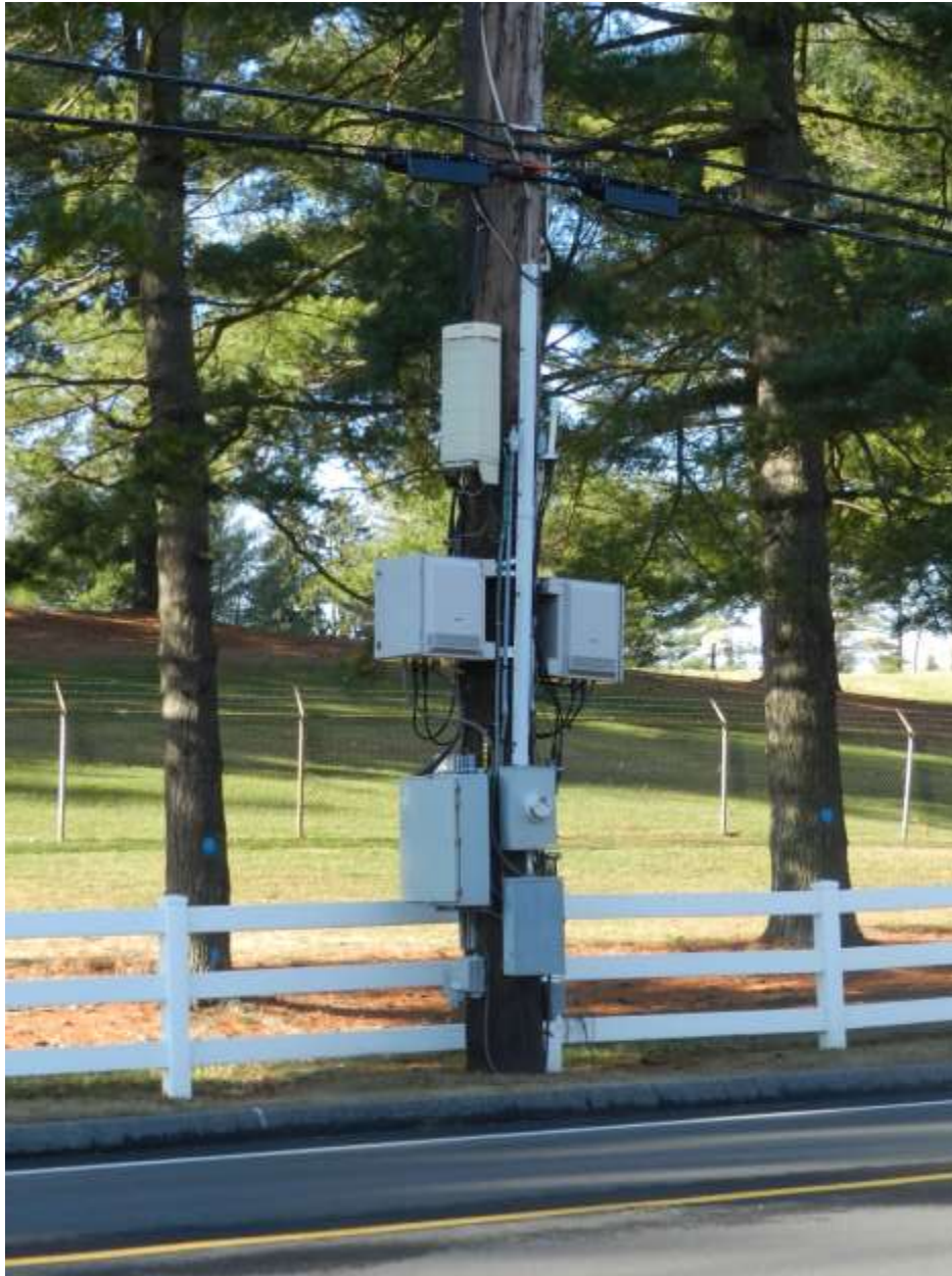
Figure 4 – Base of DAS Installation With Multiple Cabinets for Radios, Backhaul, and Power
