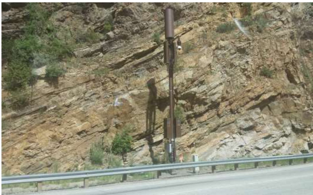
Figure 11 – Distributed Antenna Installation on U.S. Route 6 in Clear Creek County, Colorado
