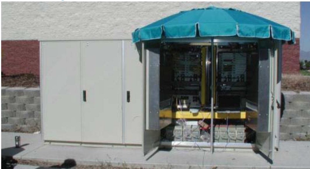
Figure 2: Fiber Distribution Cabinet (Active Ethernet Architecture)
