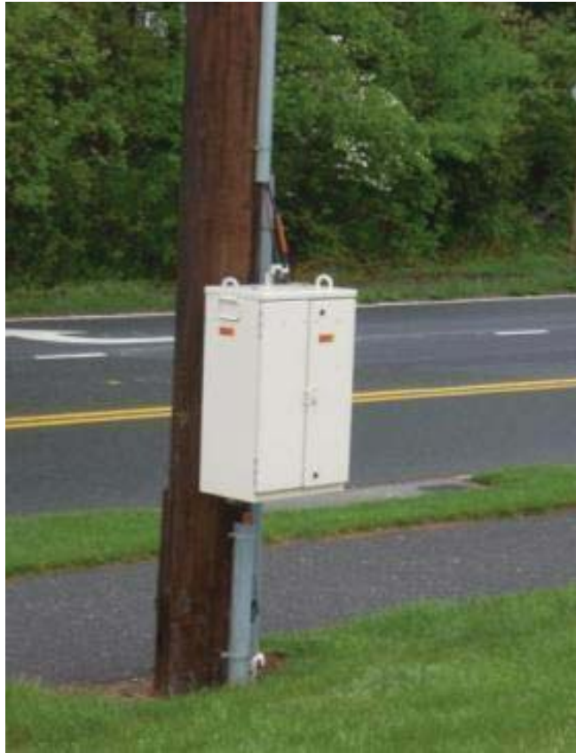
Figure 1: Fiber Distribution Cabinet (PON Architecture)
