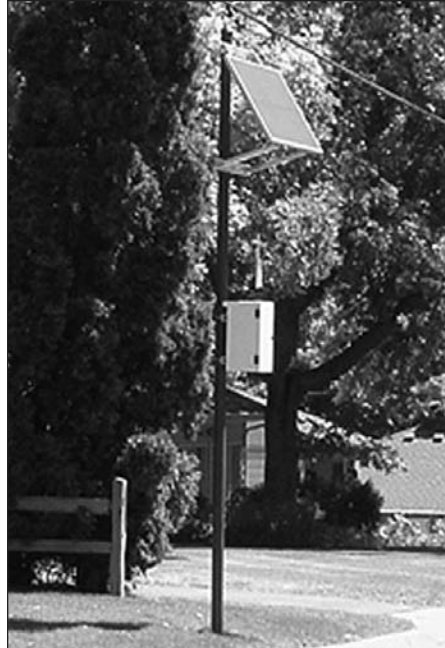
A solar-powered wireless access point on a newly installed pole.
